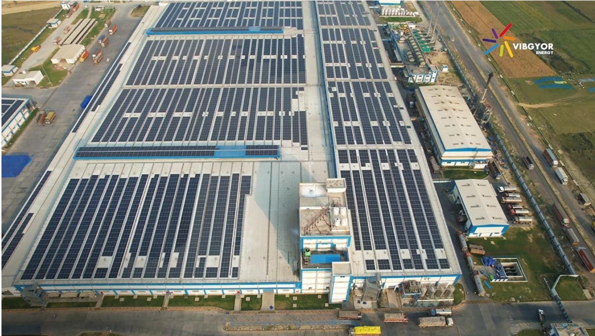
Varun Beverages · Gorakhpur, Uttar Pradesh — one of India's larger single-roof C&I solar installations.
