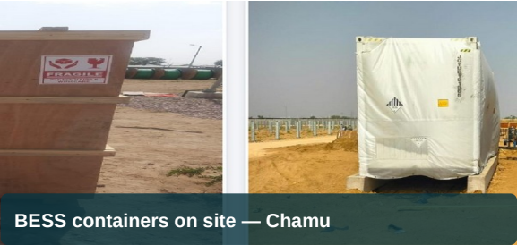
Vibgyor's 7.5 MWh battery — built for Chamu
