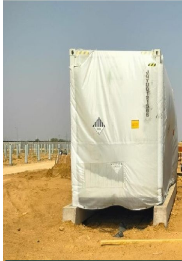
BESS containers delivered
